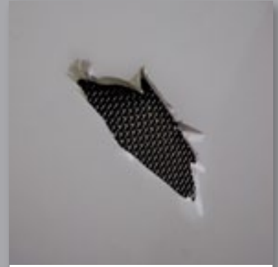
3 Cut a piece of Aluminium mesh to the approximate size of repair. Secure the mesh in place ready for the filler application.
