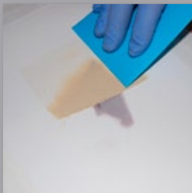
8 Then apply a full coat of ProWorx bulk filler with the applicator provided making sure that firm and even pressure is being applied.
